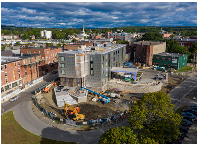
As the only hotel in downtown Waterville, the Lockwood Hotel is expected to make a significant positive economic impact in the area.
