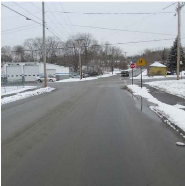
Waterville: On High Street looking west towards Drummond Ave. intersection, undersized STOP sign
